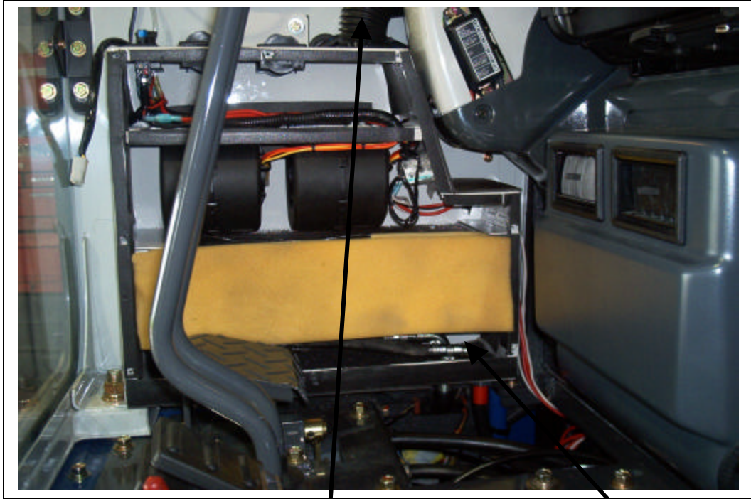
Flex hose to vent behind operator
